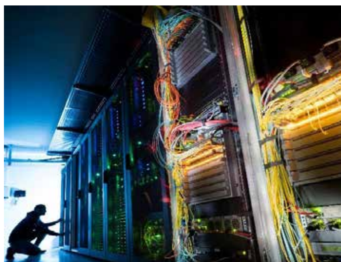
The server rooms at European XFEL; home to the facility's scientific data
