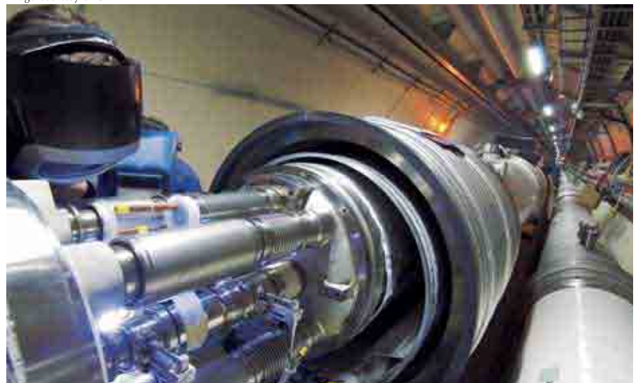
A welder making the very first interconnection between two cryomagnets for the LHC. The 1700 interconnections between superconducting magnets for the whole collider required 123 000 separate welding and assembly operations
